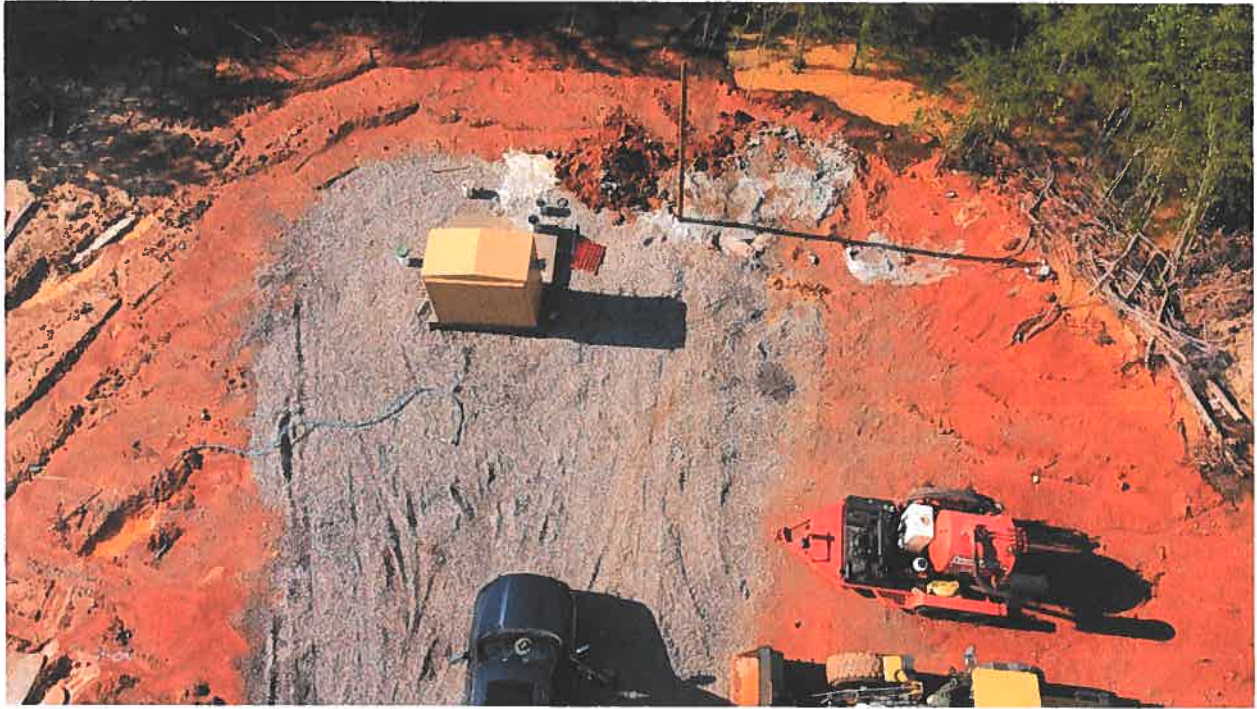
Coordinates 33.5895°, -86.1561° This is located on McCaig road near Lohr. The generator to be install on the right side of the lift station.
