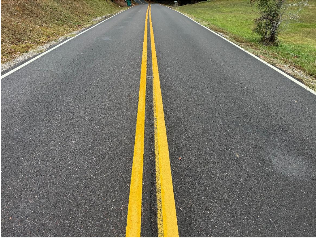
Figure 8. Example of Both Mixes at One-Year Inspection (Rubber on Left, Control on Right)
