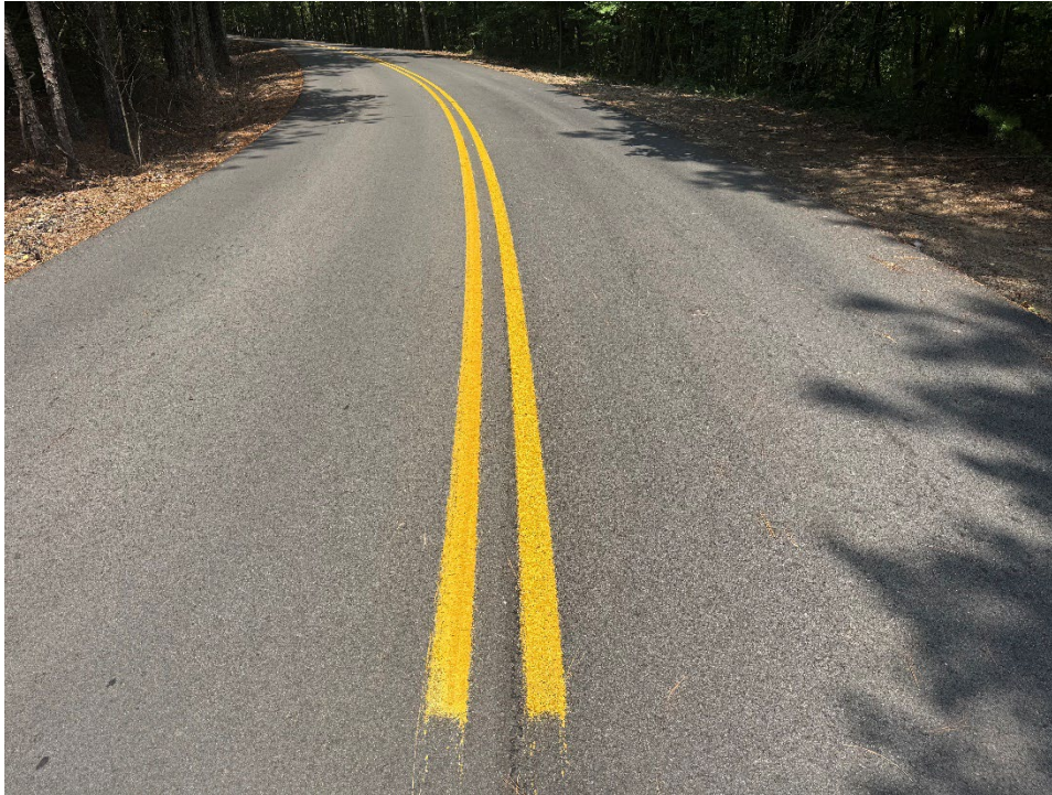
Figure 1 Example of Both Mixes at One-Year Inspection (Rubber on Left, Control on Right)
