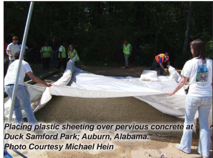
Surface Raveling; Auburn, Alabama
