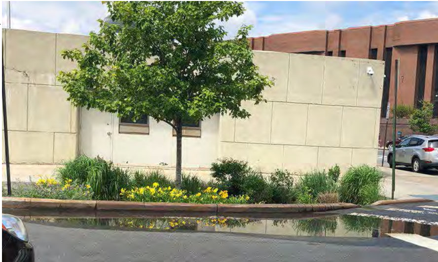
Poor grading allows water to build up on the road adjacent to a bioretention practice.
