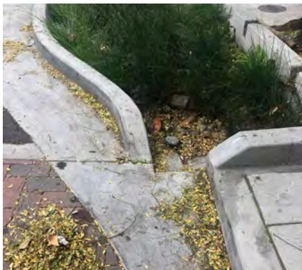
Curb Extension Inlet (Rhea Thompson)
