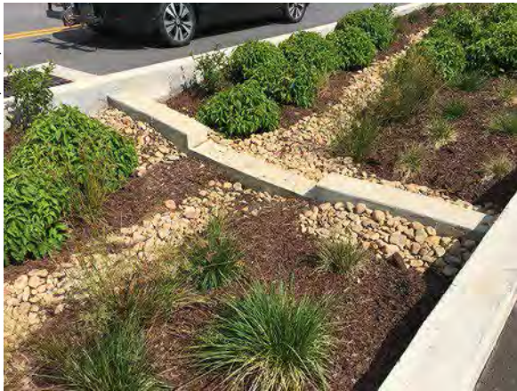
Check dam in a bioretention facility in Atlanta, GA.
