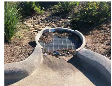
Inlet Sump Forebay (Rhea Thompson)
