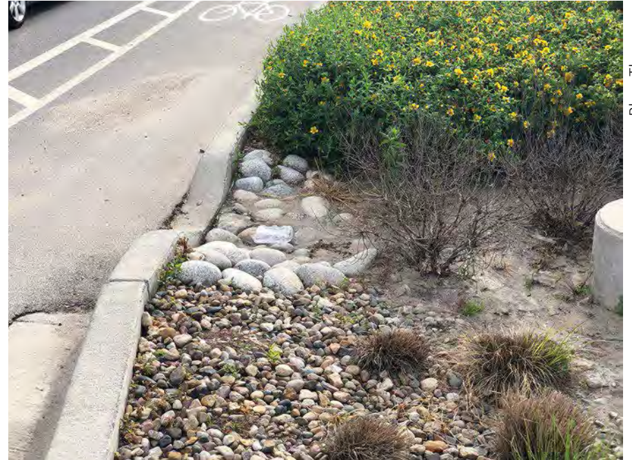
A sediment-clogged stone forebay.
