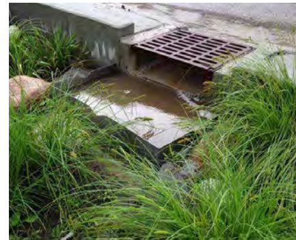
Curb Well Forebay (City of Omaha)
