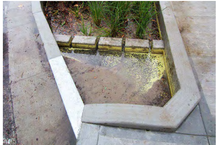
A concrete pad in a stormwater curb extension system in Portland, OR.
