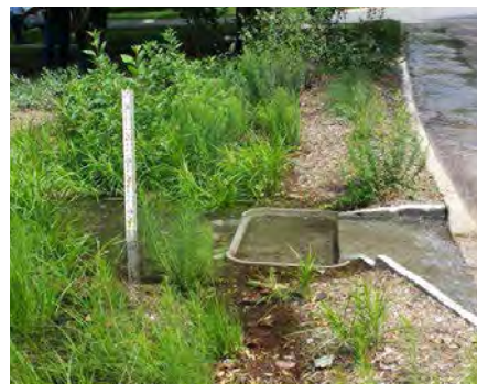
Utility Box Forebay (City of Omaha)
