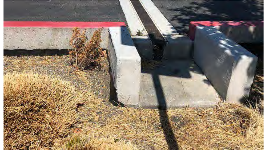
Concrete splash pad in San Mateo, CA
