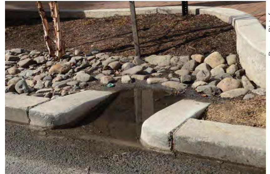
Incorrectly installed inlet.
