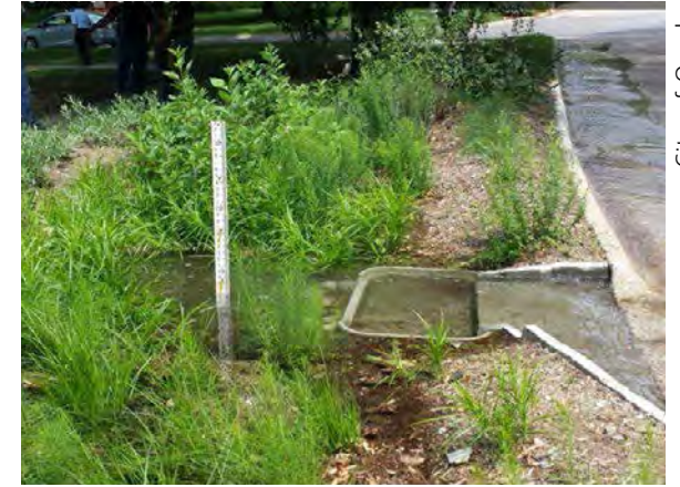
A utility box forebay in Omaha, NE.
