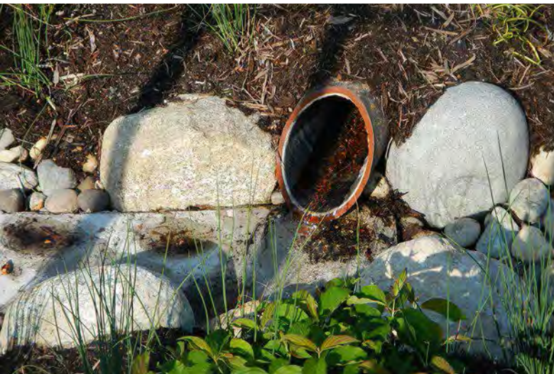
A pipe discharges runoff over an energy-reducing concrete splash pad in Seattle, WA.
