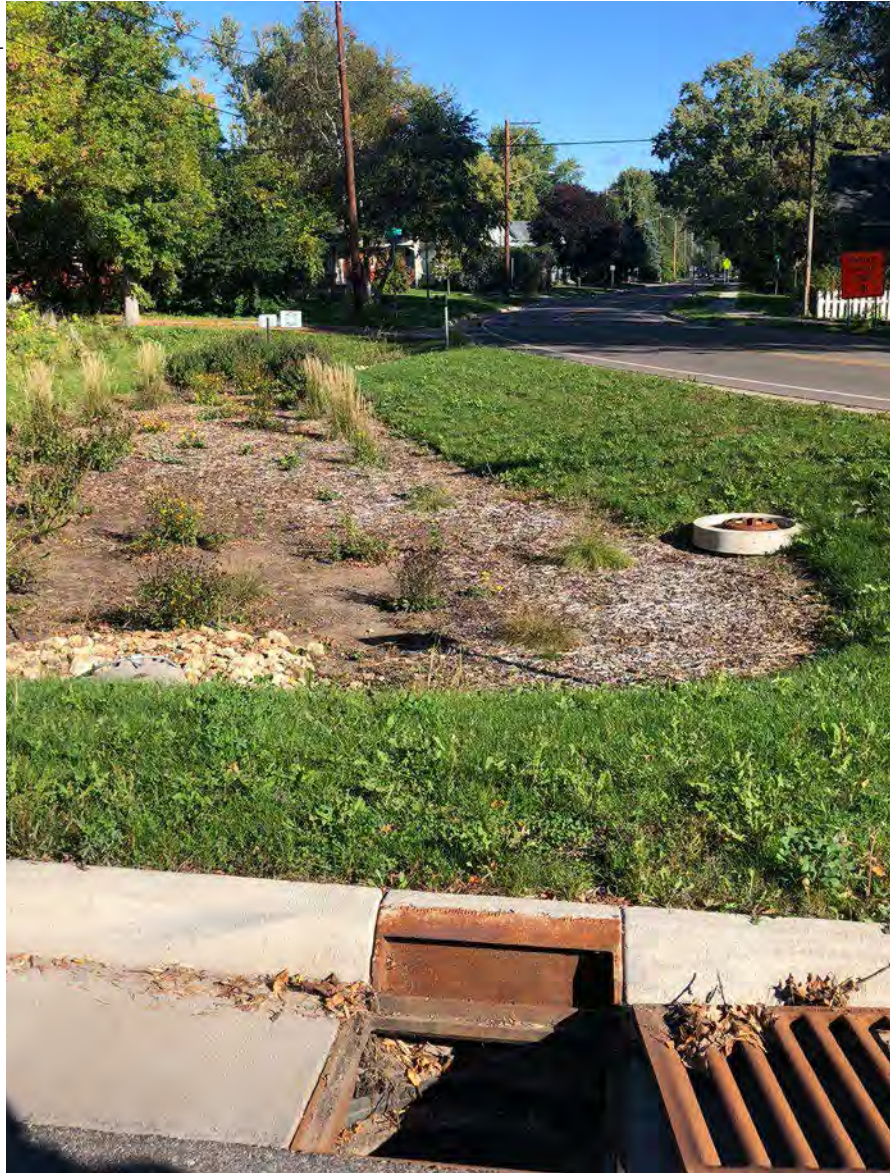
Water flows into a depressed drain and through a pipe to a bioretention facility in Minneapolis, MN.
