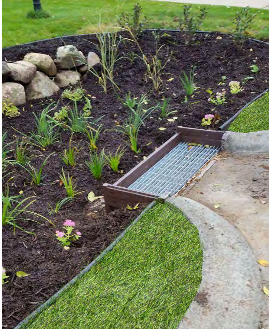
A bioretention practice in Minneapolis, MN, with a proprietary inlet sump often used in residential areas.
