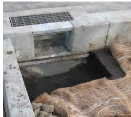
Depressed Drain (Portland Bureau of Environmental Services)
