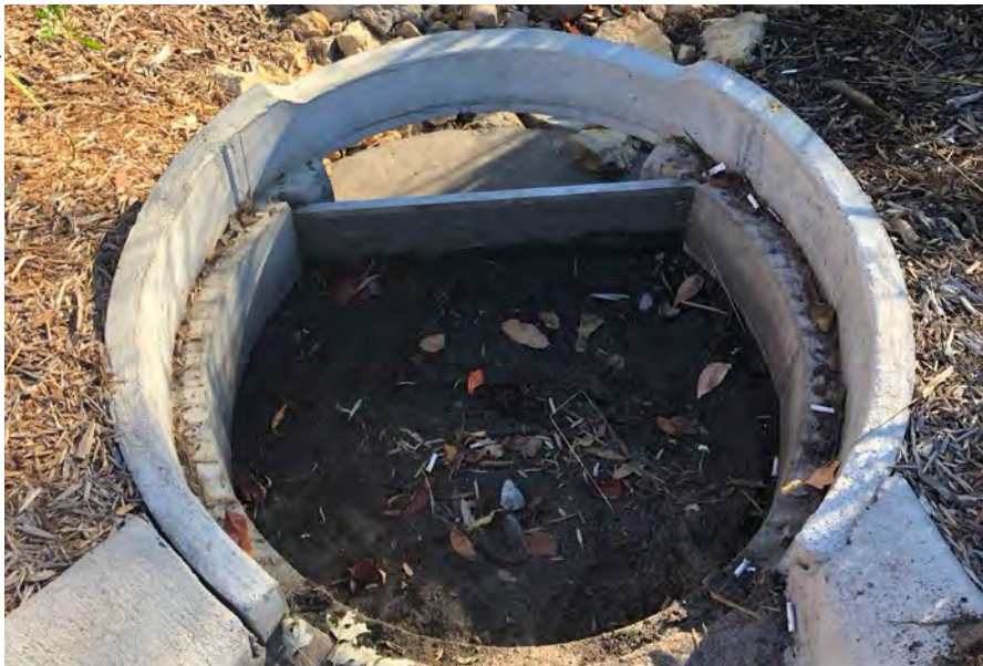
Pretreatment maintenance often requires removing the grate and scooping out sediment and debris for disposal off-site.
