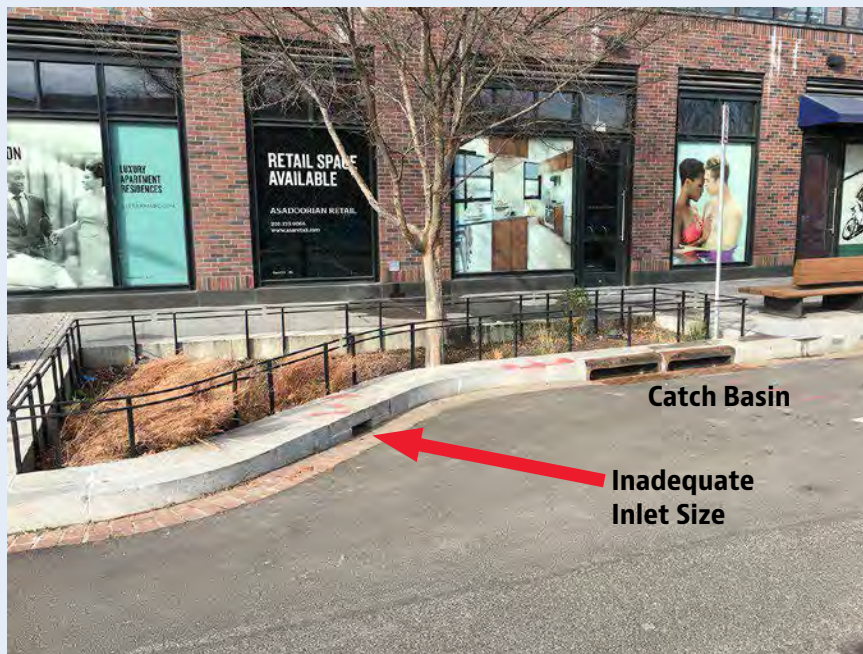
Example 1. Arrow shows an undersized, poorly functioning inlet.
