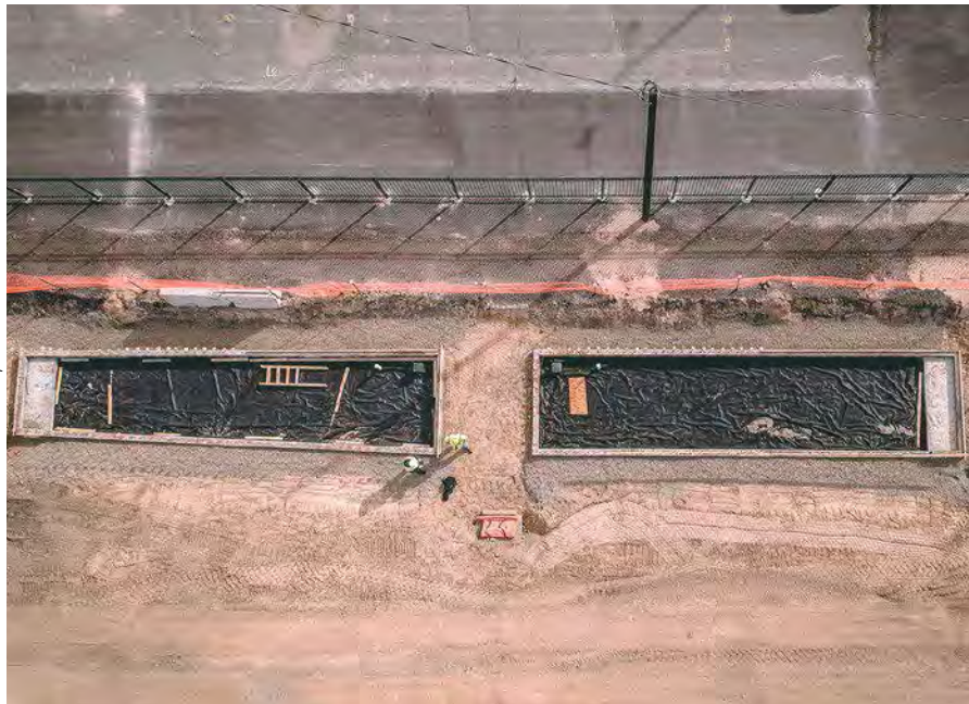
Aerial image showing impermeable liners at the bottom of two bioretention cells under construction in Denver, CO.
