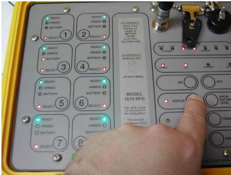
Figure 4-13 Manually checking STATUS
