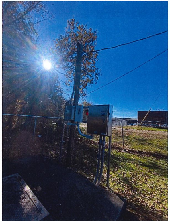
Photo #8 – Windrush Pump Station (Facing West)
