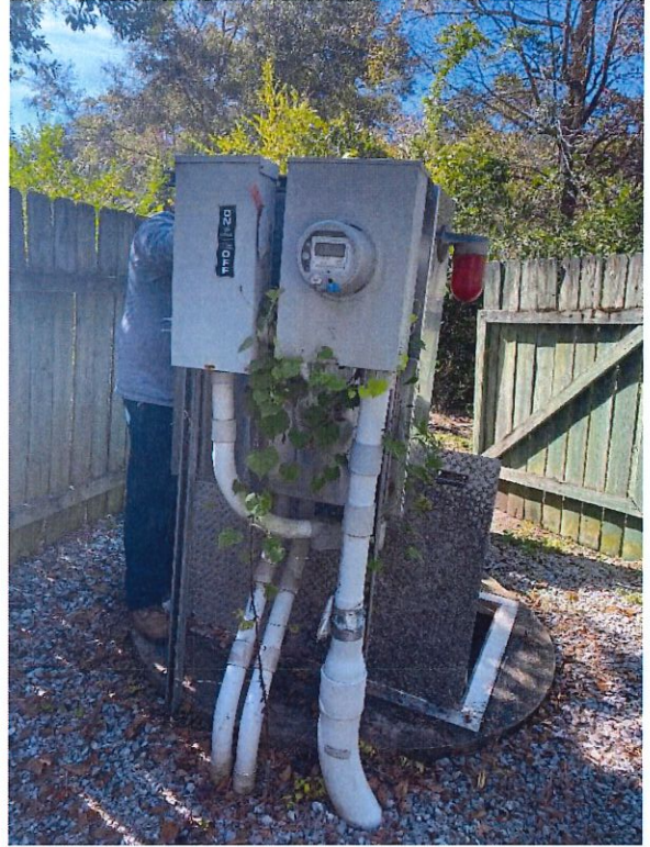
Photo #19 – Golfview Pump Station (Facing West)
