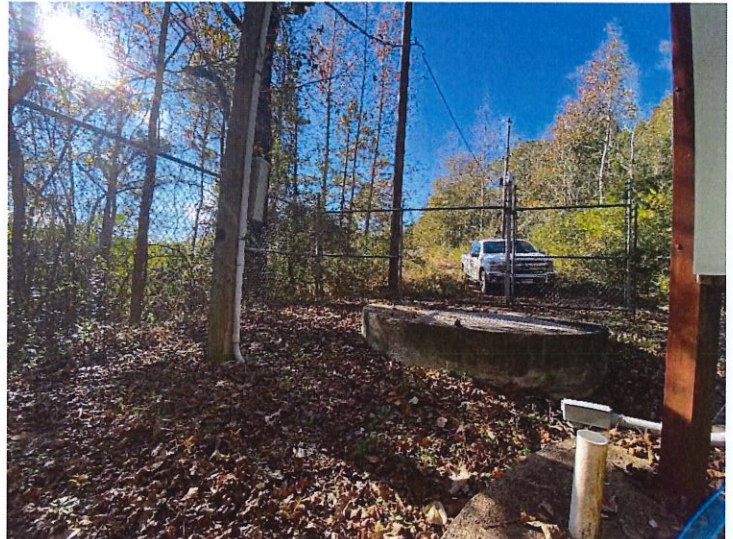
Photo #3 – Walmart Pump Station (Facing West)
