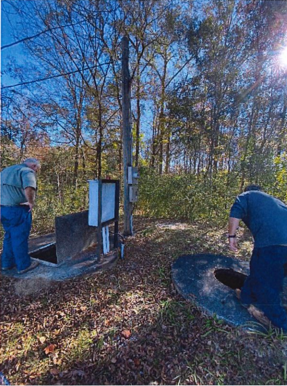
Photo #17 – Clolinger Road Pump Station (Facing South)
