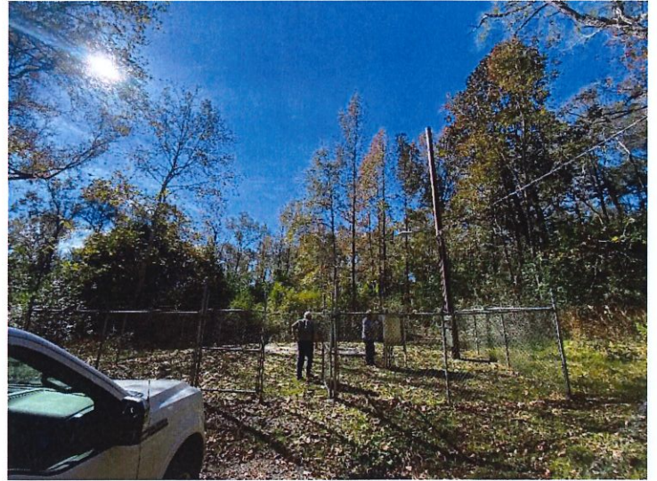
Photo #23 – Davis Pump Station (Facing Southwest)
