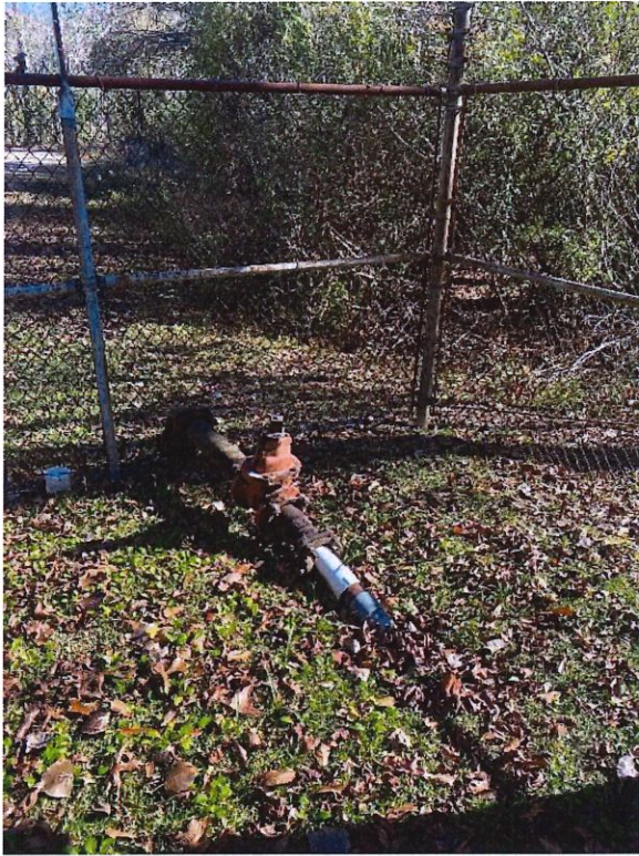
Photo #21 – Roy's Mill Pump Station (Facing Northeast)
