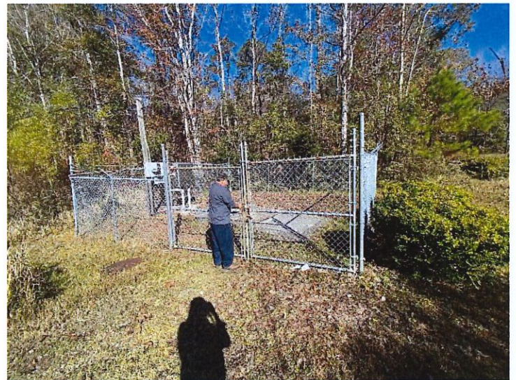
Photo #12 – Napoleon Street Pump Station (Facing East)
