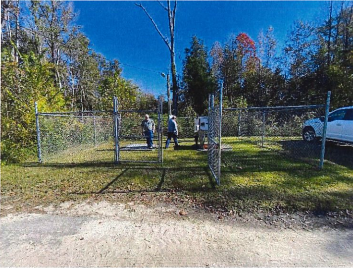
Photo #25 – Willis Pump Station (Facing East)
