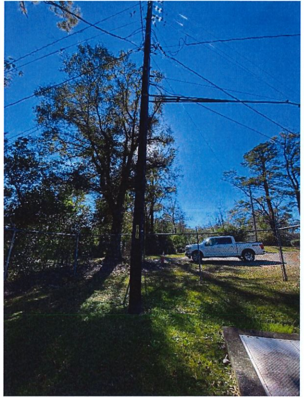
Photo #15 – Church Street Pump Station (Facing South)
