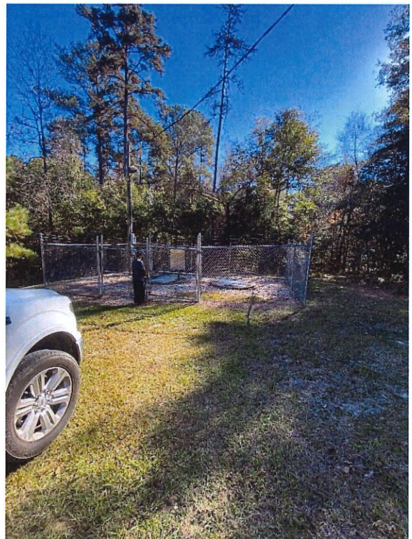
Photo #4 – Hampton Inn Pump Station (Facing South)
