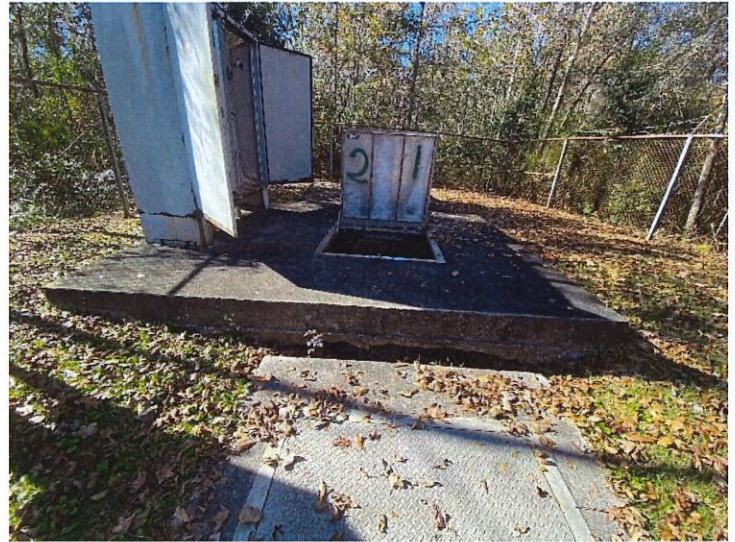
Photo #20 – Roy's Mill Pump Station (Facing Southwest)
