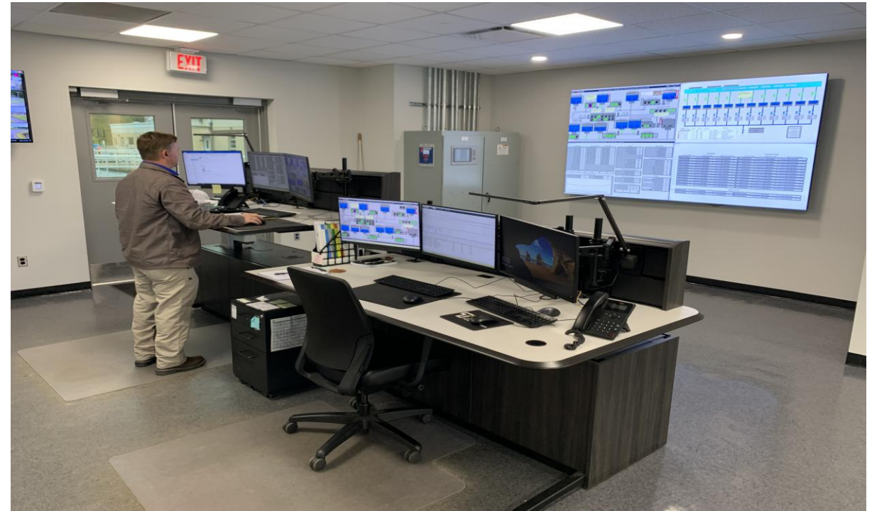
Secured control room
