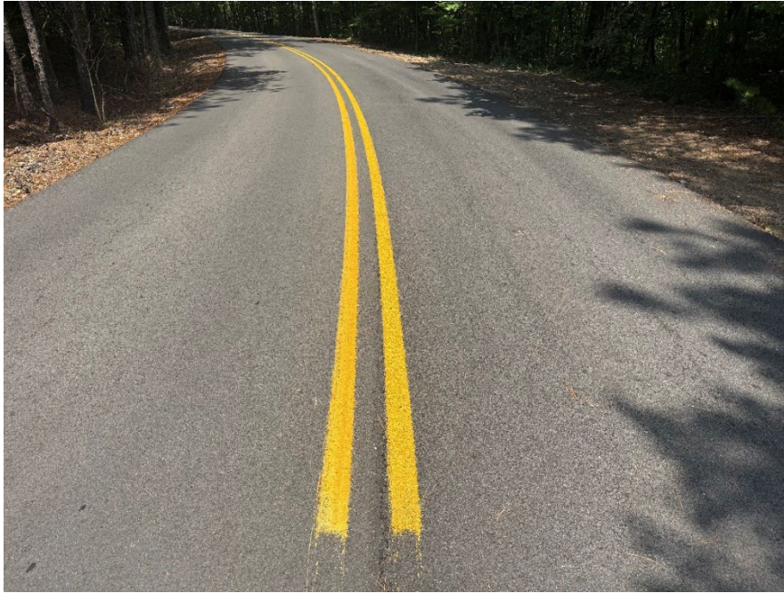
Figure 3 Example of Both Mixes at One-Year Inspection (GTR on Left, Control on Right)
