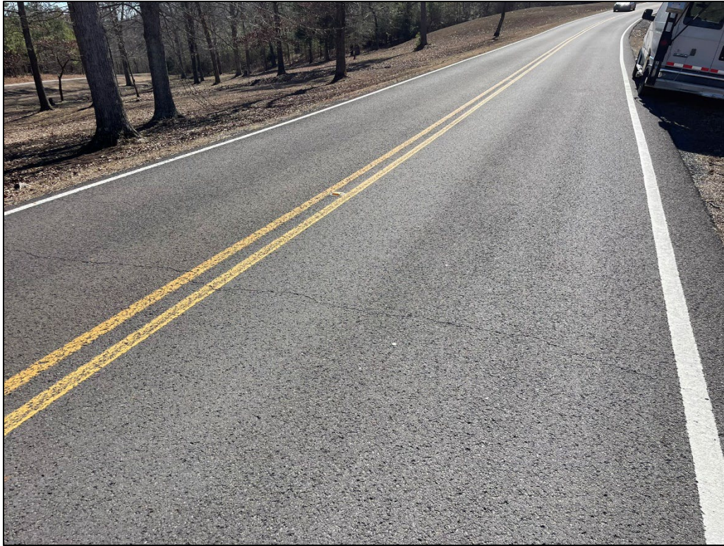
Figure 5. Example of Cracking Observed at the 2024 Survey
