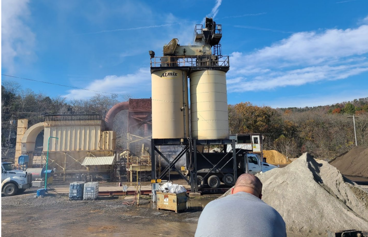
Figure 1. WCC Plant near Guntersville, AL
