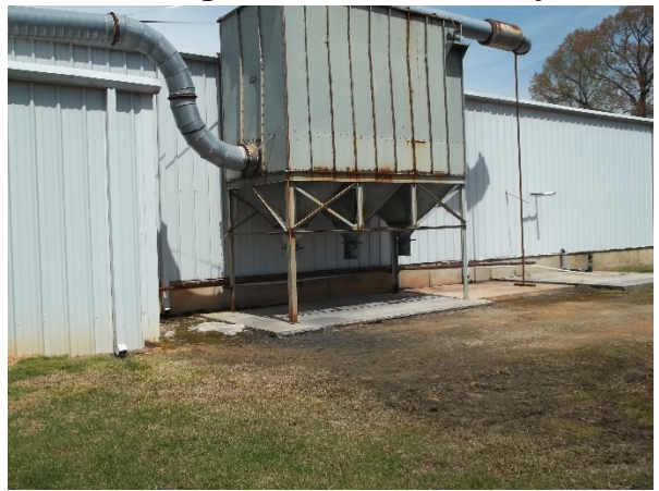
Baghouse at the Facility
