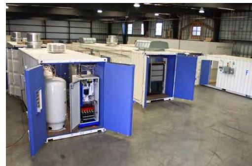
Custom 200 ppd ozone sparge system - prove out
