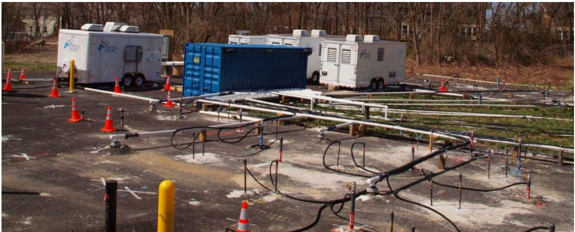
Ozone, SVE and air sparge systems installed at site.
