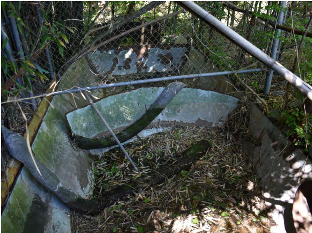
Photo No. 32: Baffled drainage basin along the west boundary.
