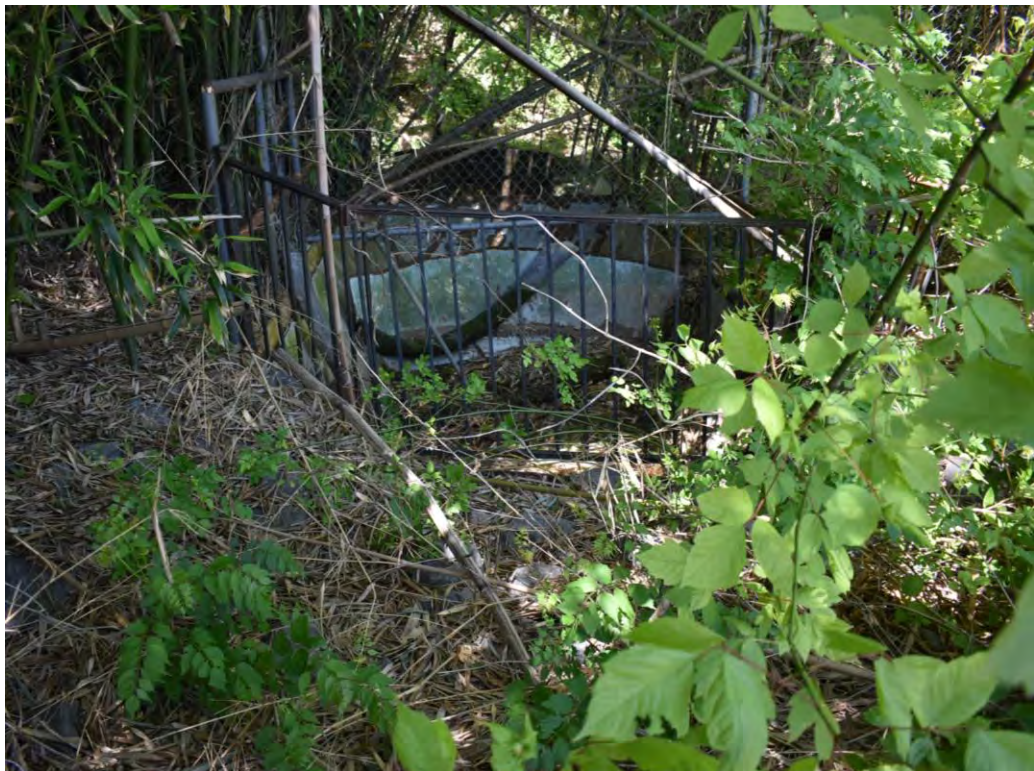
Photo No. 30: Stormwater retention basin along the west-central property boundary.
