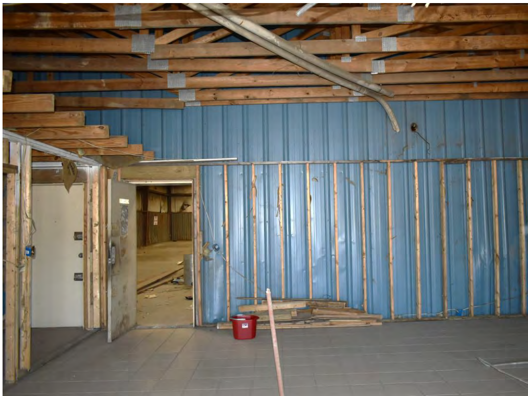
Photo No. 43: View from the south structure to the warehouse portion of the building.
