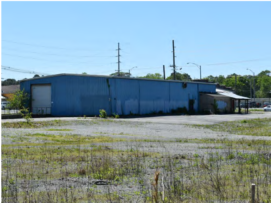
Photo No. 27: View of the west side of the structure from the northwest portion of the subject property.
