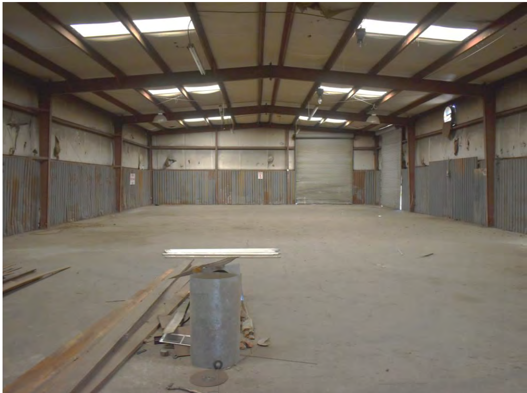
Photo No. 44: View north of the interior of the warehouse portion of the building.
