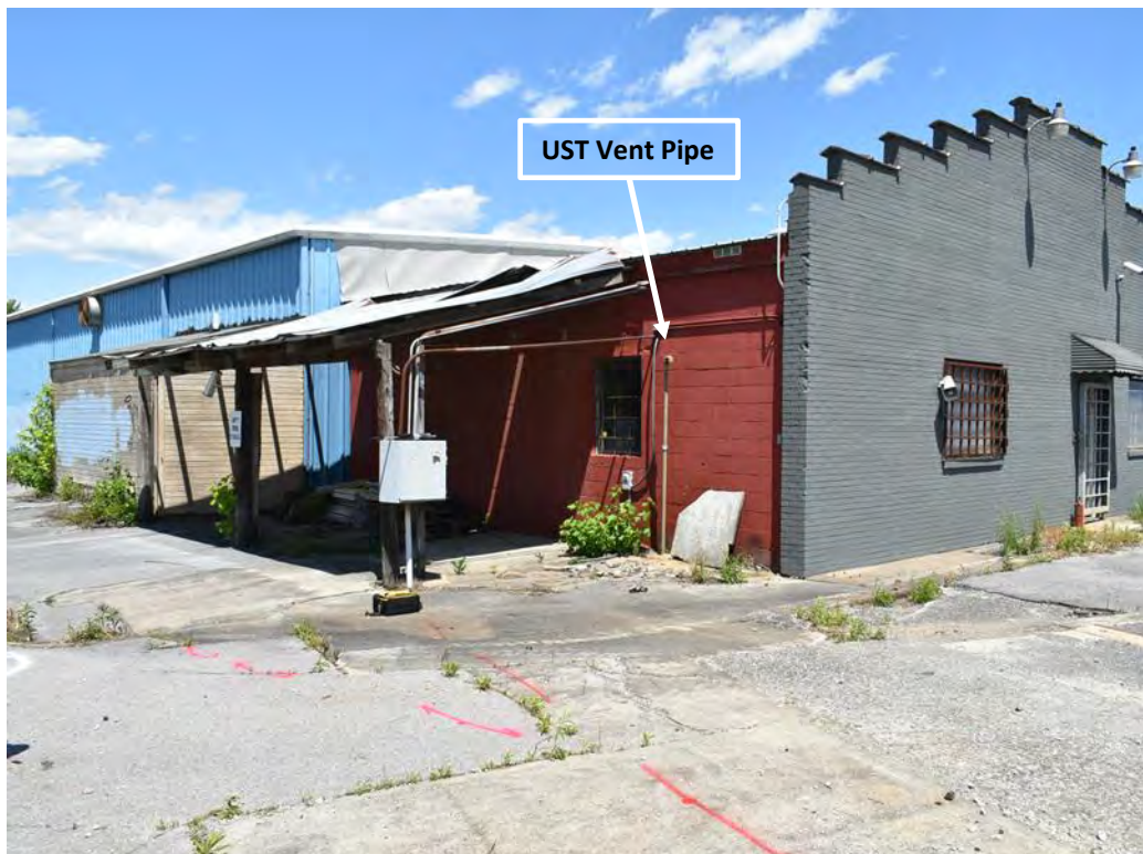
Photo No. 38: Former UST and drum storage area on the southwest corner of the building.
