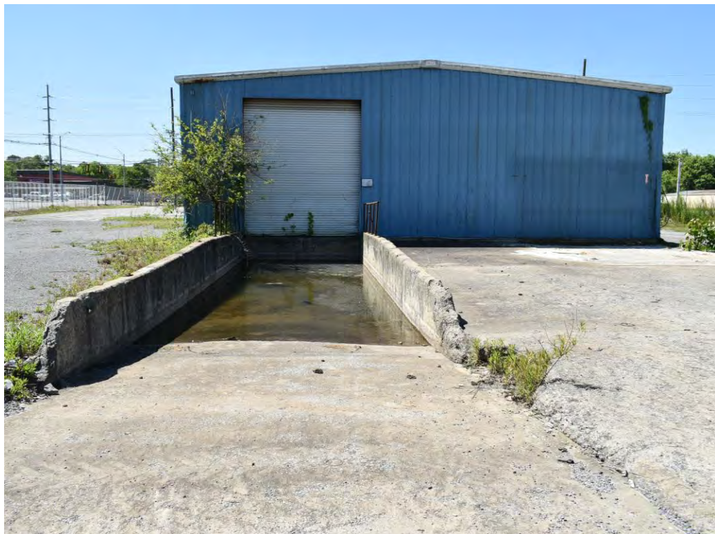
Photo No. 16: View of the loading dock and concrete pad on the north end of the structure.
