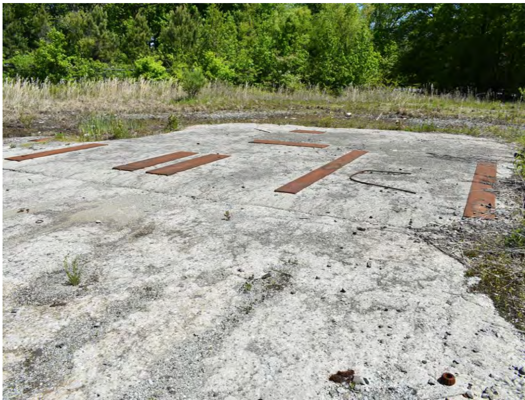
Photo No. 23: Concrete pad in the north portion of the subject property where materials were scrapped.
