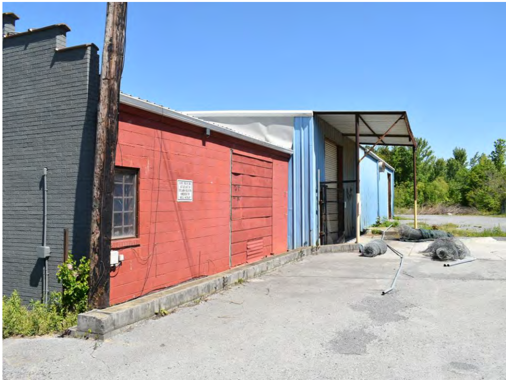
Photo No. 6: View north from the northeast corner of the structure on the subject property.
