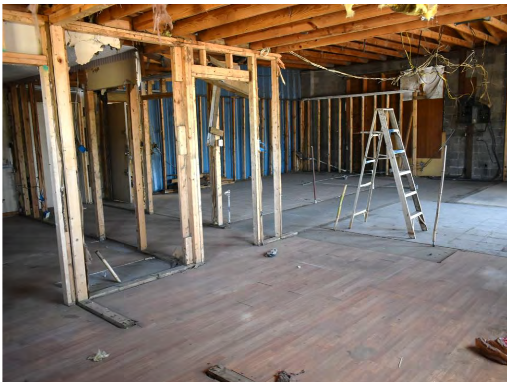
Photo No. 42: Additional view of the interior of the south portion of the structure.
