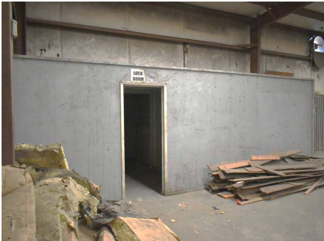
Photo No. 46: Interior storage and restrooms in the southwest corner of the warehouse.
