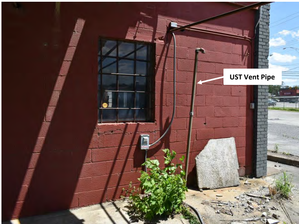
Photo No. 39: Vent pipe for a UST that was reportedly removed circa 2000.
