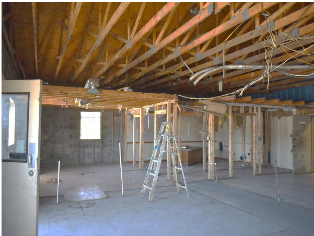
Photo No. 41: View of the interior portion of the south end of the structure.
