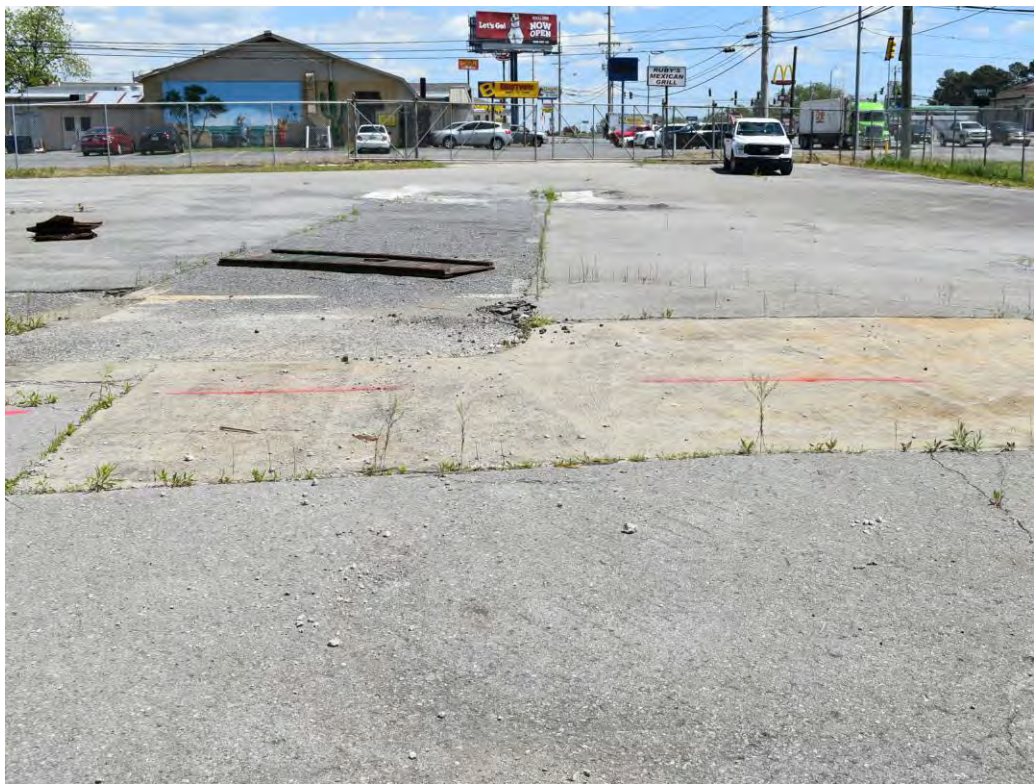
Photo No. 37: Former weigh scale along the south side of the building.
