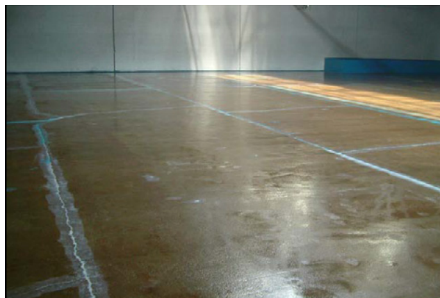
Completed surface preparation consisting of shot blasting, Retro-Coat PREP, to fill joints and cracks and a 6 mil application of Retro-Coat PRIMER
