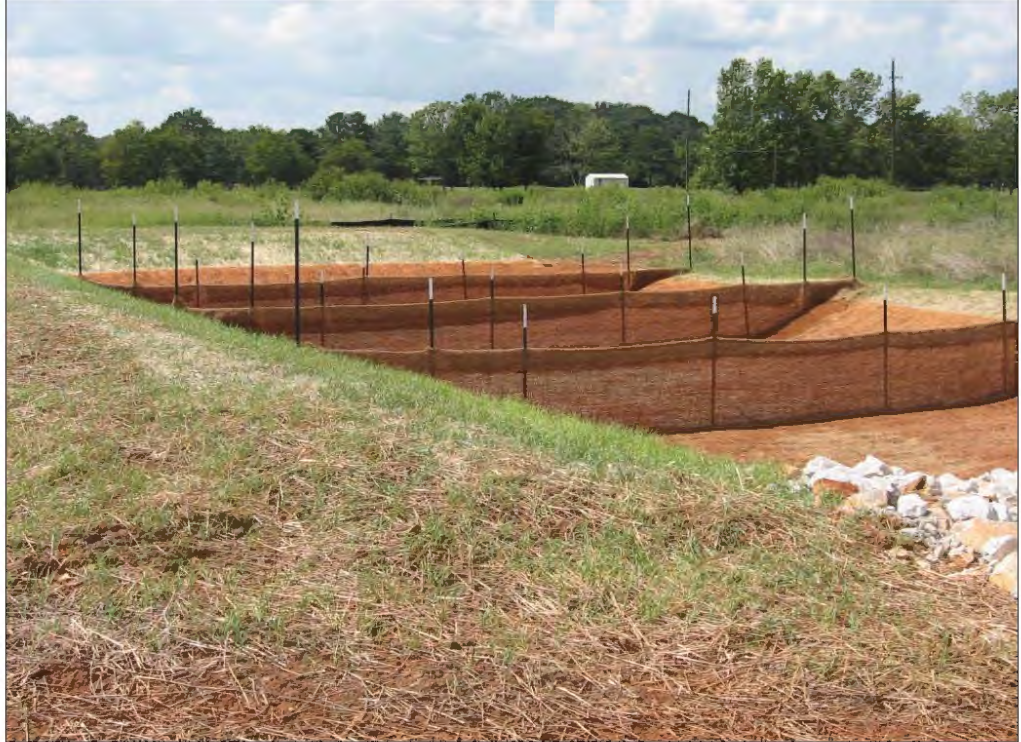
Example of porous baffle made of 700 g/m 2 coir erosion blanket as viewed from the inlet
