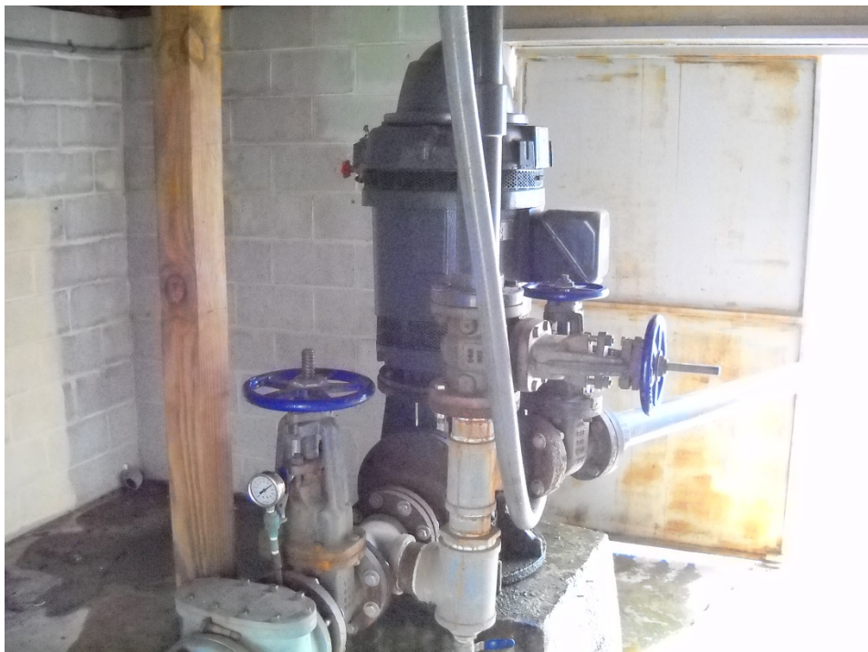
On-site production well formerly used in pump and treat system
