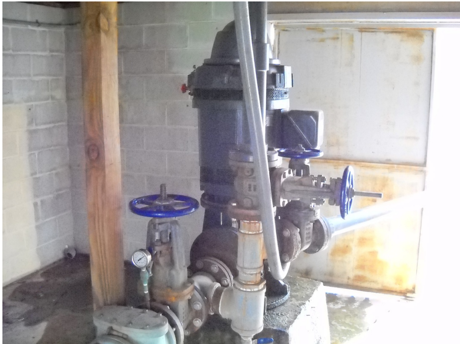
On-site production well used in pump and treat system
