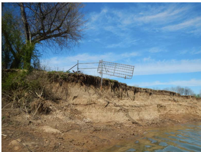
Fig. 12. Eroded bank at CABB-7, on Lower Cahaba River, downstream of Centreville, Alabama, March 19, 2019. Photo by Cal Johnson.
