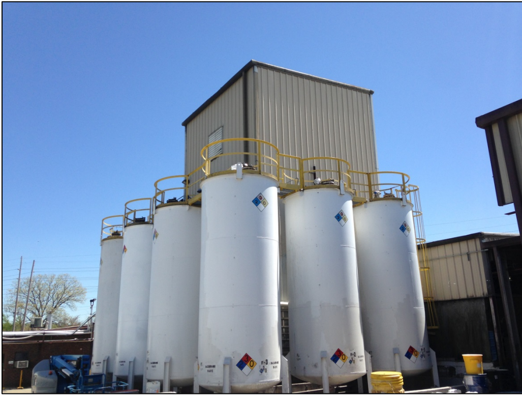
Tank System 2—Southeast View
