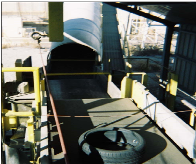
Automated feed system for introduction of scrap tires into the kiln at the Lafarge Building Materials, Inc. cement plant, Calera, Alabama.
