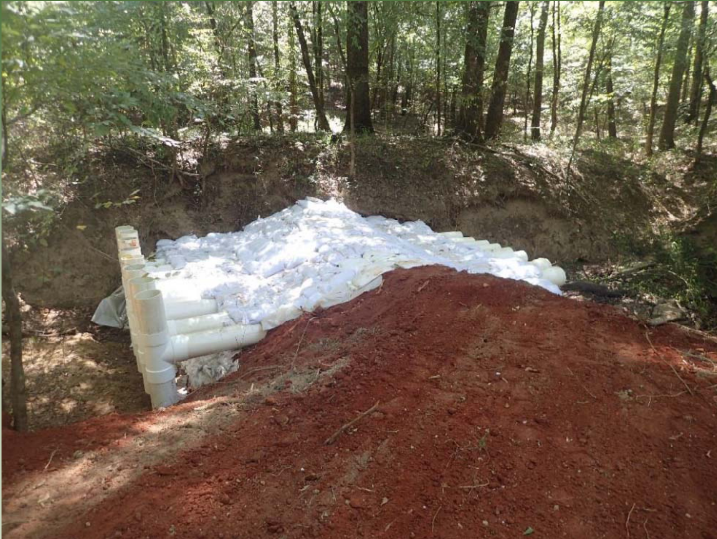
Completed underflow dam in Peel Creek, approximately 200 feet southeast of the Cahaba River
