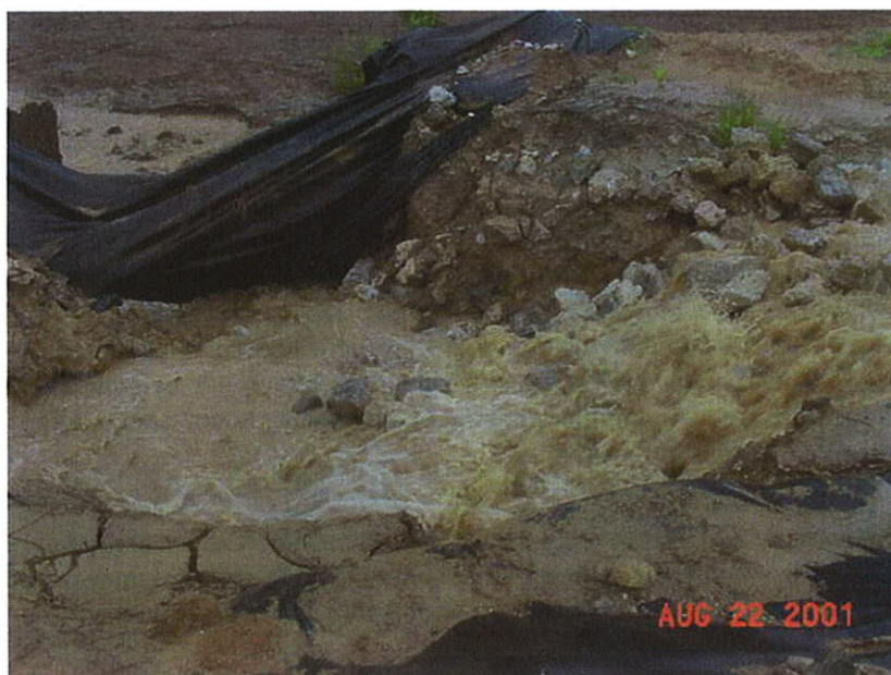
Photo 1: Improperly installed silt fence
