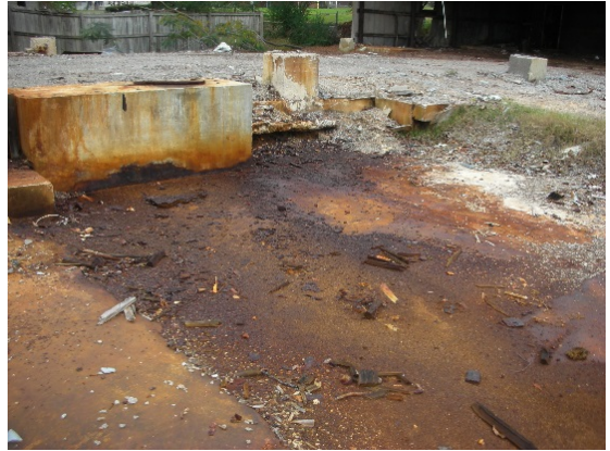
Stained Foundation Area
