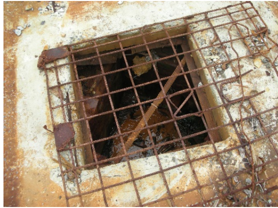
Underground Drainage Pipe
