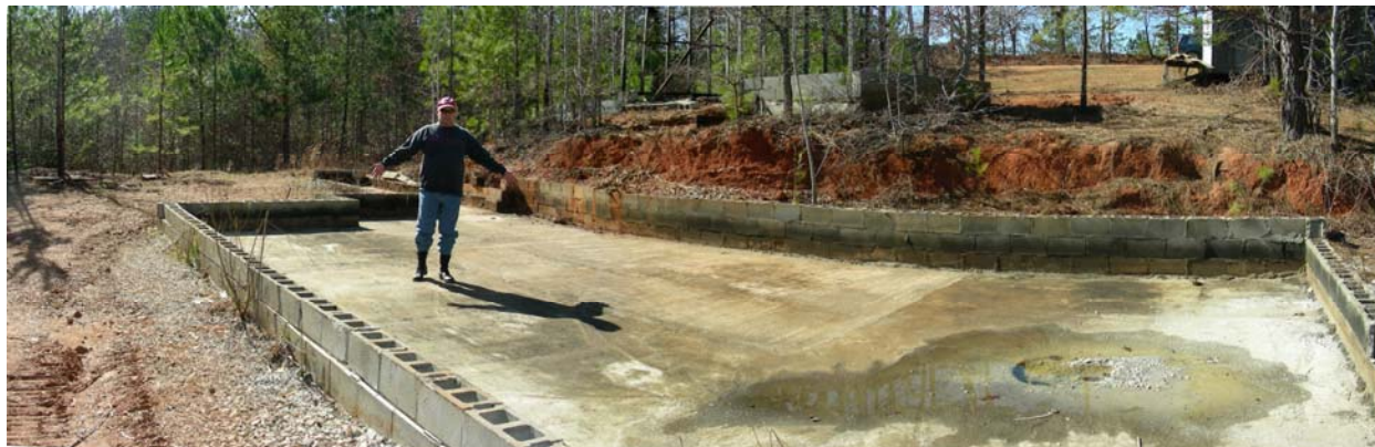
Secondary Containment for Former Above-Ground Storage Tanks Holding Waste Oil at McCullough Oil Recycler, Verbena, AL
