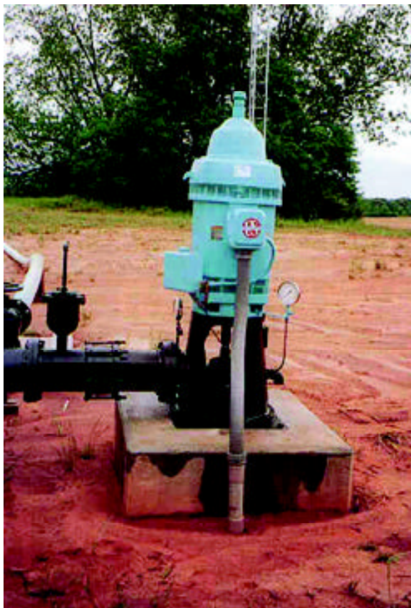
The Mount Carmel public water supply well in Pike County is the deepest in Alabama, at 2723 ft.
