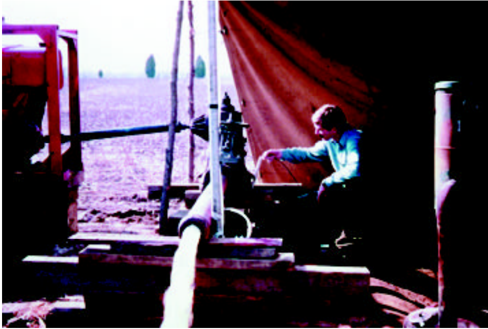
A pump test can reveal how much water an aquifer can yield to a well.
