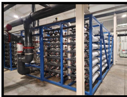
PFAS Removal System
